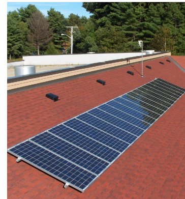
Solar panels on Shutesbury Elementary School earned through
